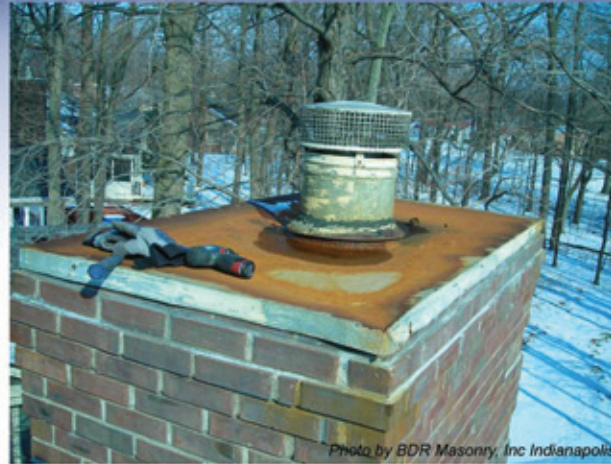
Chase is rusted and no longer functioning correctly or safely.
